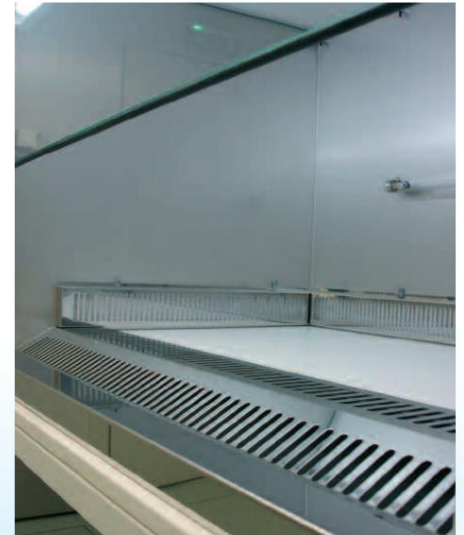
Pre-filter on return
